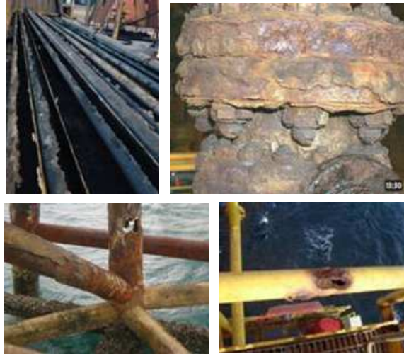
Figure 2 – Corrosion of mature installations tubing corroded by CO 2 - Surface valve - Corroded structure- Hole in a railing
